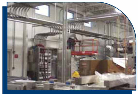
Conduit Racks in the Process Side of the Plant
