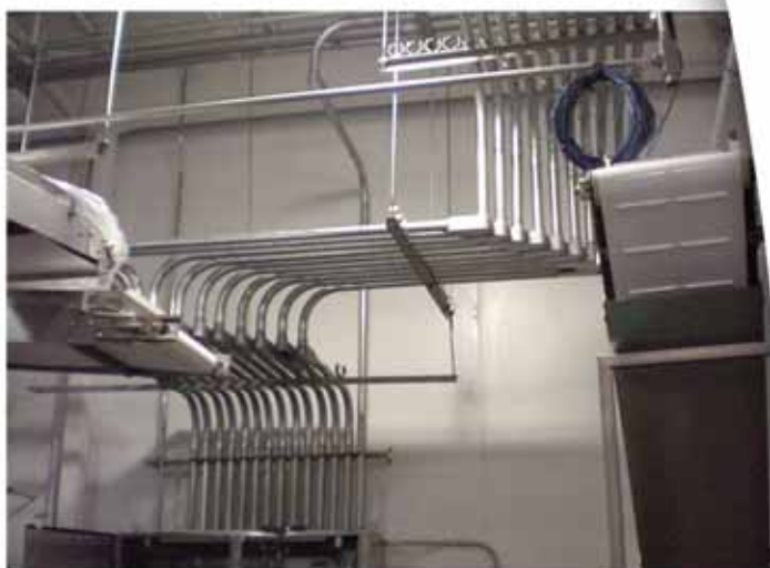
Conduits from Production Line Panels
